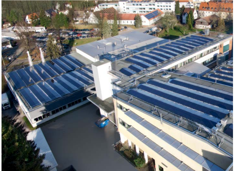
Photovoltaic system on E-T-A's roof
