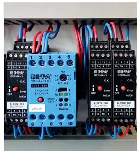
Replacing old by new: E-1072-128-DC 24 V-3A and E-1071-128-DC 24 V-3A
